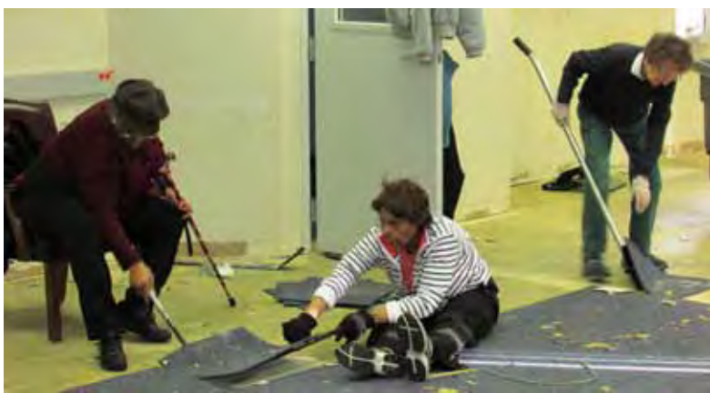
Citizens Police Academy alumni assist in the demolition at the new police station.
