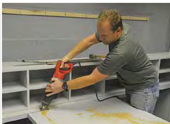
South Holland Lions member Roger Bonnema helped with removal of old work stations.
